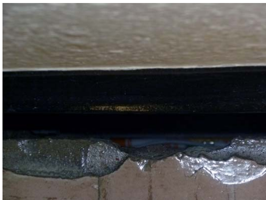
Figure 2 -Floor of Annex separating from structural wall – one of several structural cracks
