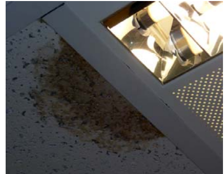
Figure 1 - Bathroom leakage from above
