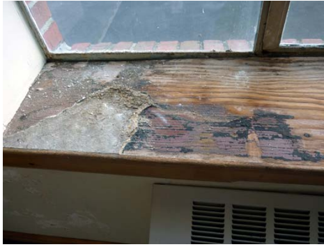
Figure 1 - Single pane window wall - leaks & energy inefficient
